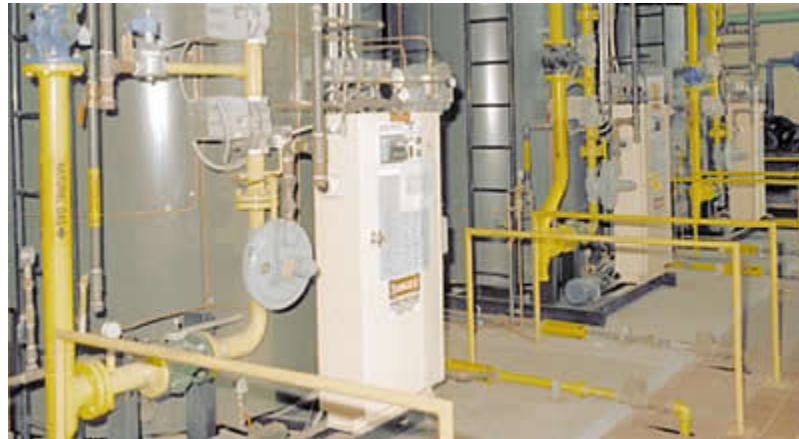
Figure 2. Steam metering at the CRC.
