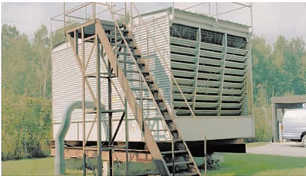
Figure 1. Cooling unit at the CRC.
