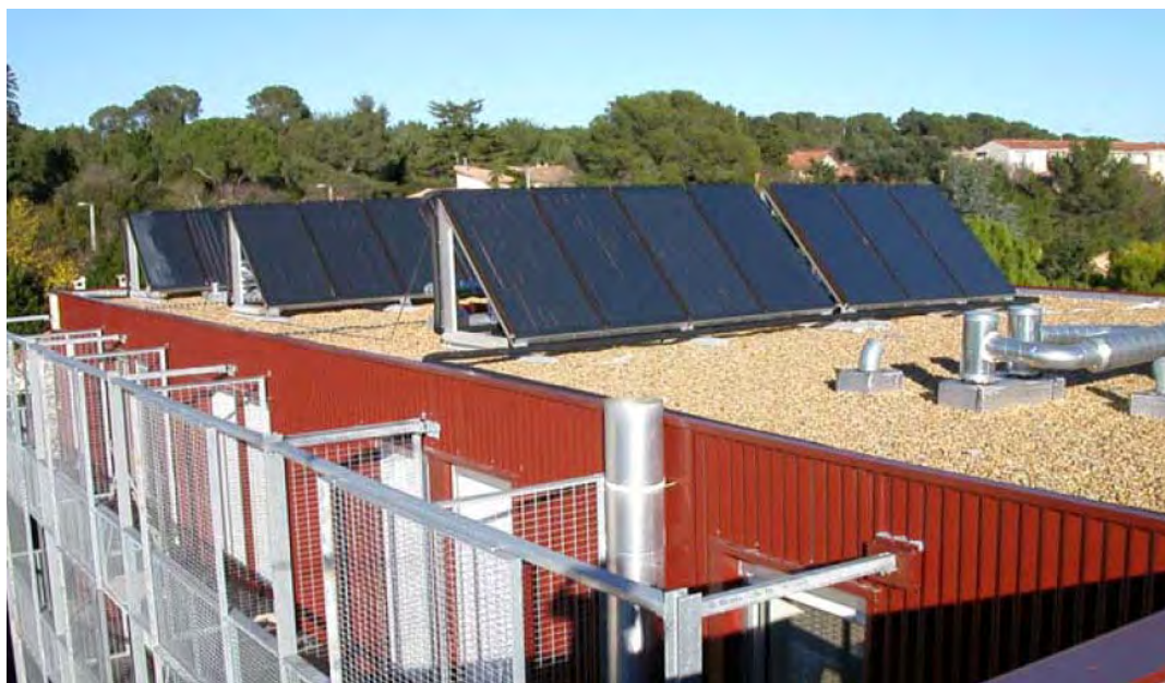
Figure 7. Solar collectors on the roof.
