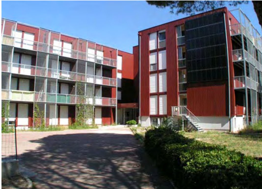
Figure 6. Outside insulated envelope.
